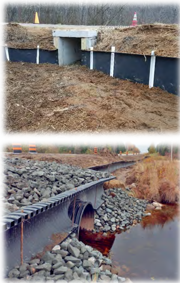
Figure D-31. Two types of small animal fences: Top, plastic drift fence-wall, bottom, half pipe barrier wall. Photo Credits: Top B. Zarate, New Jersey Division of Fish and Wildlife, Bottom, taken from Heaven et al. 2019, Ontario.
