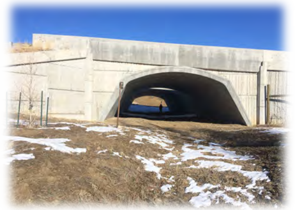
Figure E-5. Monitoring camera is placed on steel post approximately 30 feet (9 meters) from entrance of structure on US 160 in Colorado. Photo Credit: P. Cramer.
