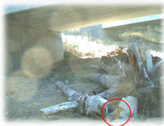
Figure 3-27. Additional small features can make the wildlife crossing structure function for smaller animals. These logs and stumps were placed under Oregon DOT's US 97 Bend wildlife crossings, and were used quickly by small mammals. Photo Credit: Oregon DOT, Oregon State University, P. Cramer.
