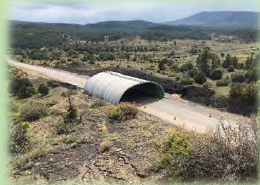
Figure A-10. Colorado US 160 wildlife overpass under construction. Photo Credit: A. Johnson.
