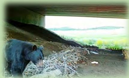
Figure A-13. A Black Bear used a new wildlife underpass on I-25. The woody material was placed along the structure for small mammals. Photo Credit: Colorado Parks and Wildlife.
