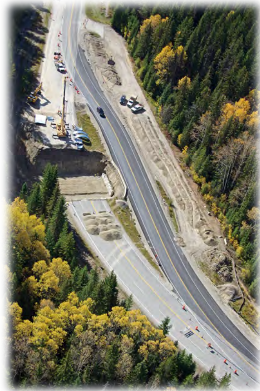
Figure 3-26. Highway 93 through Kootenay National Park in Alberta Canada received the “Kootenay Pond” wildlife underpass in 2015. A 23 x 13 feet (7 x 4 m) corrugated steel pipe (culvert) was placed under three lanes of highway. Traffic was re-routed to one side of the highway. The detour and a former parking area to the right were later decommissioned and restored. Photo Credit: Parks Canada.
