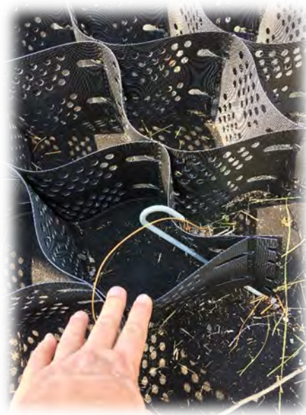
Figure D-34. Erosion control webbing was used to potentially deter animals from entering fenced right-of-way. Photo Credit: P. Cramer.
