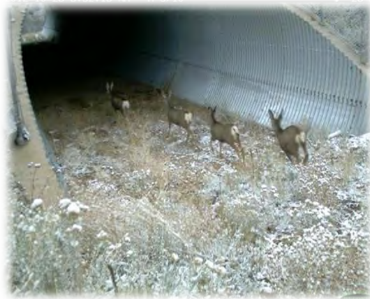
Figure D-26. In Utah, mule deer use a large corrugated steel culvert underpass in Deer Creek State Park under US 189. Photo Credit: P. Cramer, Utah DOT.
